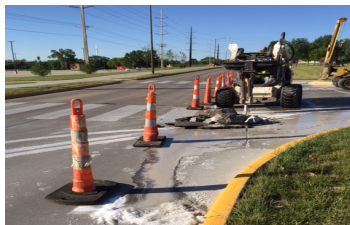
Absorbent gel used to contain wet saw cuttings. Vacuums can be used as well.
